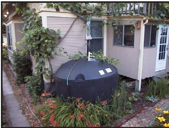
Figure 6.12 Residential Cistern. Source: Shockey Consulting Services
