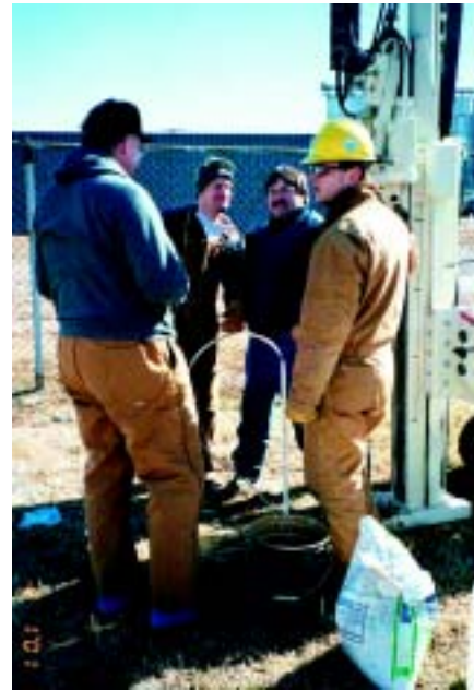
Staff install a direct-push well for temporary or permanent long term monitoring.
