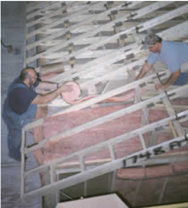
Employees of Taylor Homes in Anderson install insulation – an essential component of an energy-efficient house. DNR photo by Kerry Cordray
