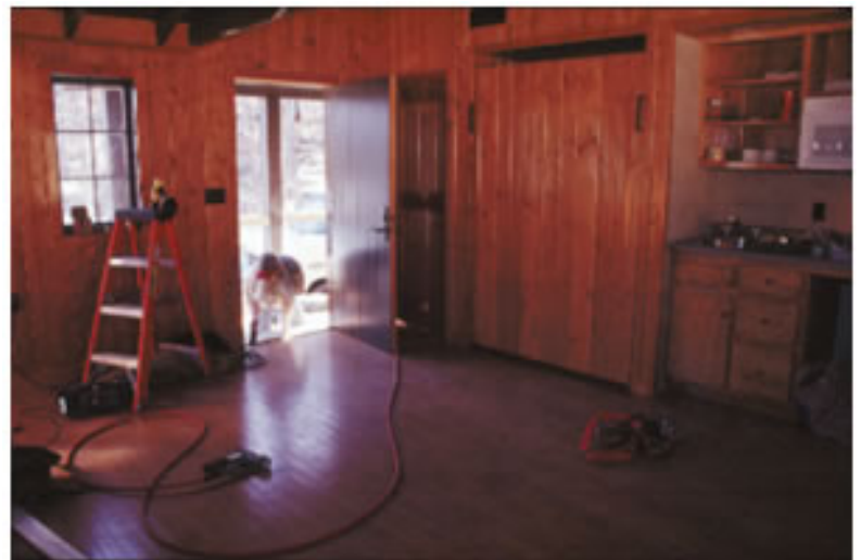
At a Civilian Conservation Corps cabin at Bennett Spring State Park, the rustic original decor has been restored from the open ceilings to the wooden floors. DNR photo by Scott Myers.
