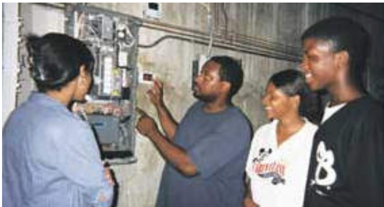
Head custodian Ron Jones of Langston Middle School in St. Louis shows some seventh-graders how the temperature control panel monitors the school's heating and cooling operations. Photo by Mid-American Energy and Resource Partners
