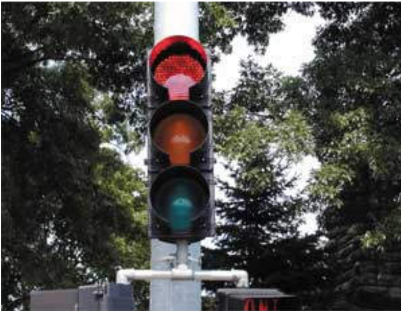
This signal head at 59th and Brookside in Kansas City is one of more than 2,500 to be fitted with 20-year 14-watt LED bulbs. The conventional bulbs only last about one year and use approximately 150 watts. Photo by Dave Buchanan / Kansas City Public Works Department
