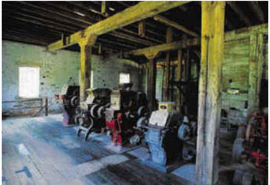
A collection of rollstands at Bollinger Mill represent the evolution of the roller milling process from the mid-1800s to the turn of the century. Only a few historic mills remain that interpret this important milling process for the general public.
