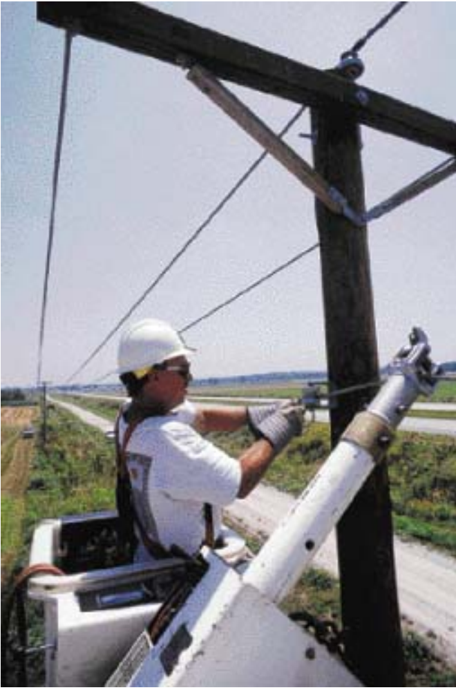
AmerenUE lineman Chip Webb replaces one of several poles damaged during a June thunderstorm. Utility competition may mean one company generates electricity while another company distributes it.
